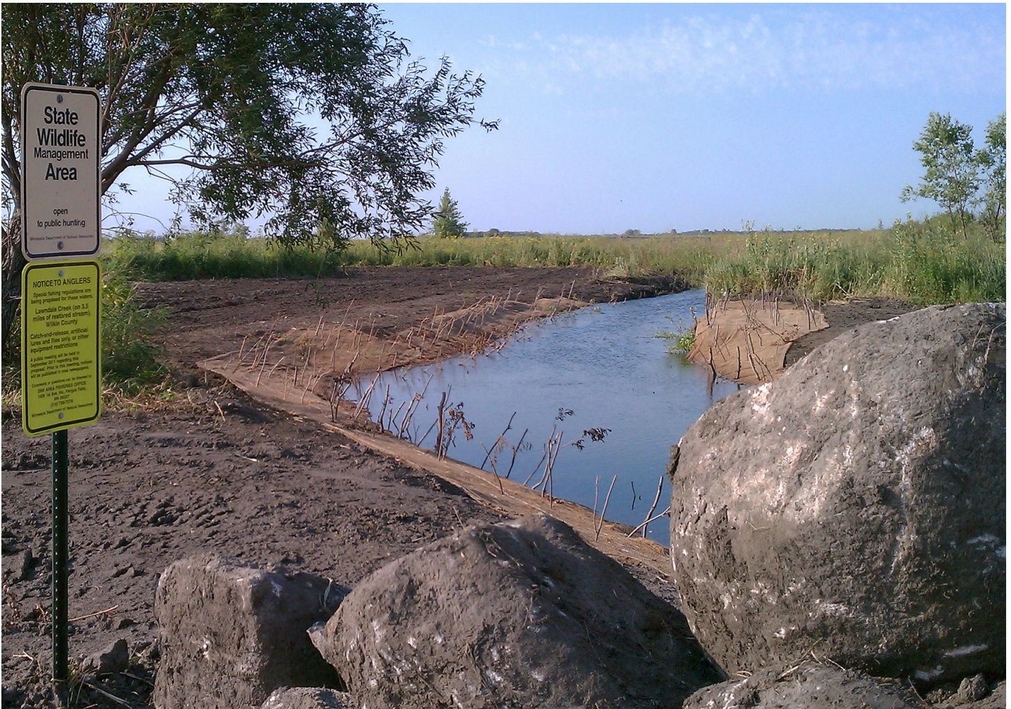
Figure 29. Local organizations restored Lawndale Creek's naturally meandering channel to reduce erosion and improve habitat in the trout stream in the Buffalo River Watershed.
