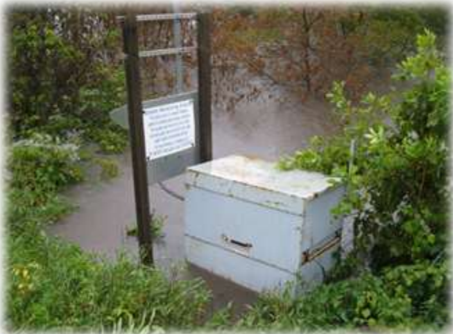
Figure 52. Beauford Ditch monitoring station, September 2010.
